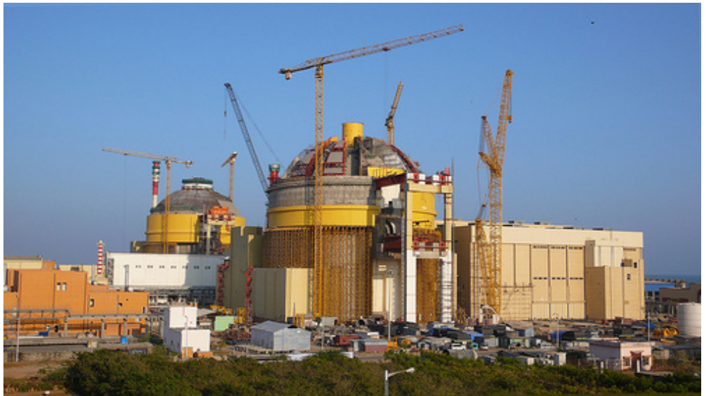
The construction of India's Kudankulam Nuclear Power Project in the state of Tamil Nadu
